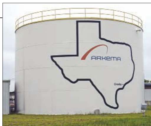
FIGURE 5. A wireless pressure transmitter was installed on this firewater tank, replacing a simple mechanical sight gauge that fails full
