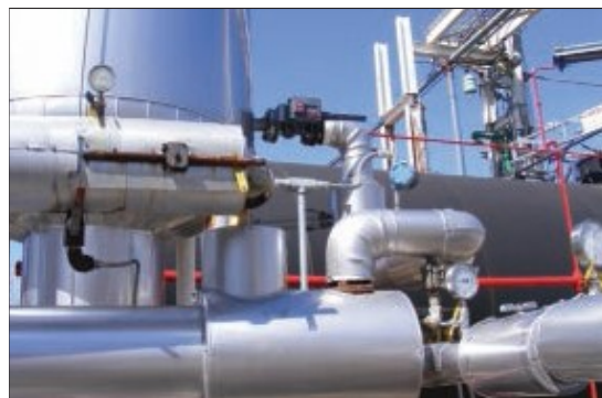
FIGURE 3. The installation of 22 wireless position monitors helped this facility save $25,000 per incident related to the release of propylene and ethylene oxides
